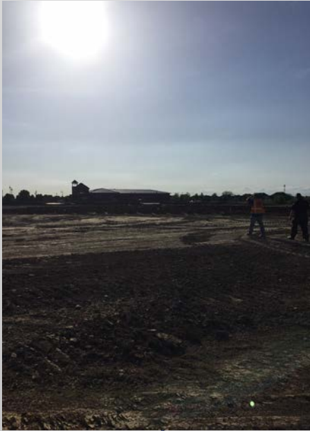
Chief Burgner getting a tour of the site and the mass grading
