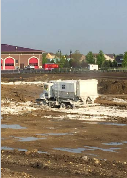
Three layers of lime were tilled into the ground bringing our pad up 2-3 feet
