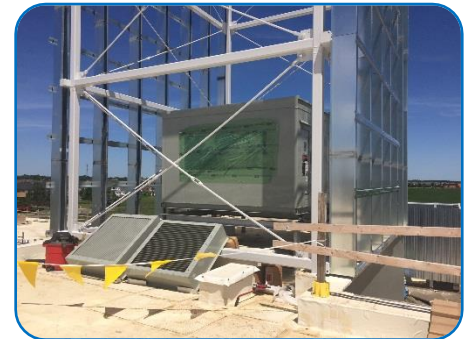
Installed Tower Unit
