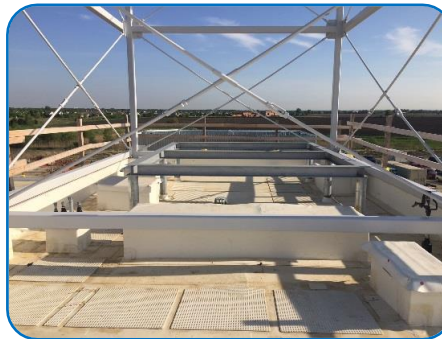
Mechanical Pad located in the Tower
