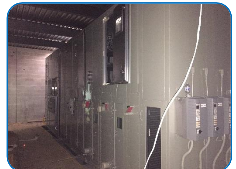
Large Mechanical Unit located in the Range Mechanical Room
