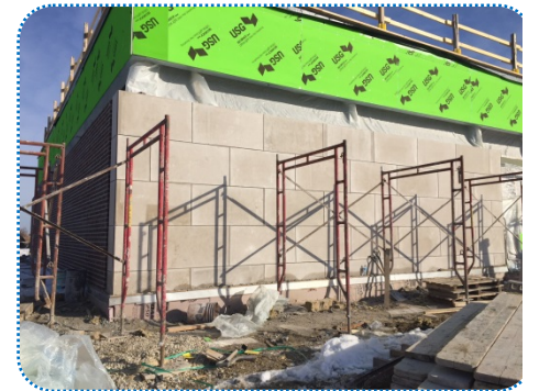
A.L.L. Masonry began installing the stone on the South Training Wing wall.
