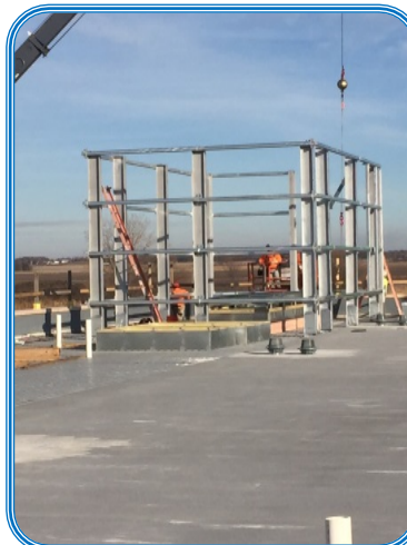
Steel walls surrounding one of the mechanical units.
