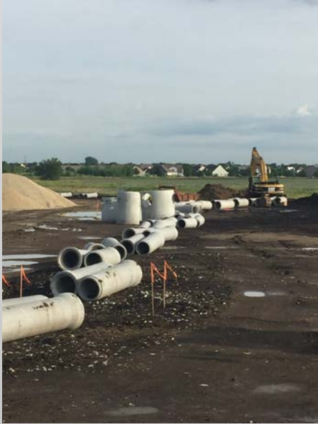
The Storm Water Detention work started this week. The pipes are lined up and ready for permanent placement.
